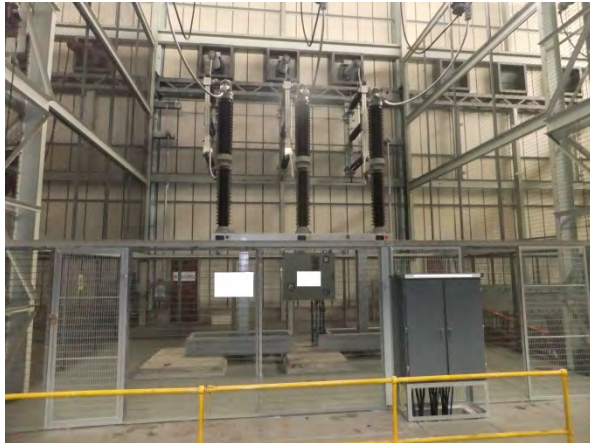
Figure 12 - Example of an utilised 132kV bay at Tottenham 132
