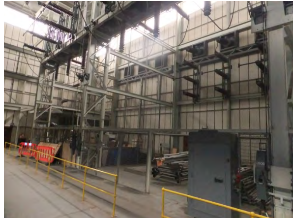
Figure 13 - Example of a spare 132kV bay at Tottenham 132 (availability/suitability to be confirmed)
